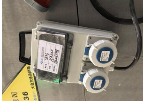
Electricity box of venue
