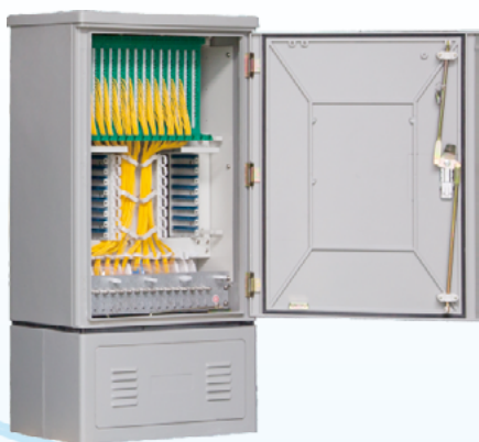
交接箱 Cross-connection Cabinet
